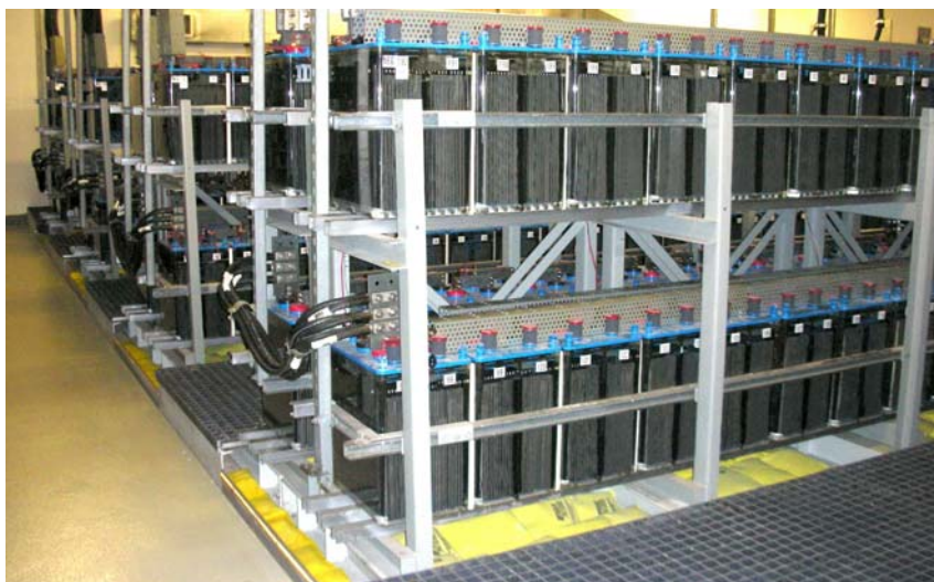
Fig 1. Typical large FLA UPS battery room.
