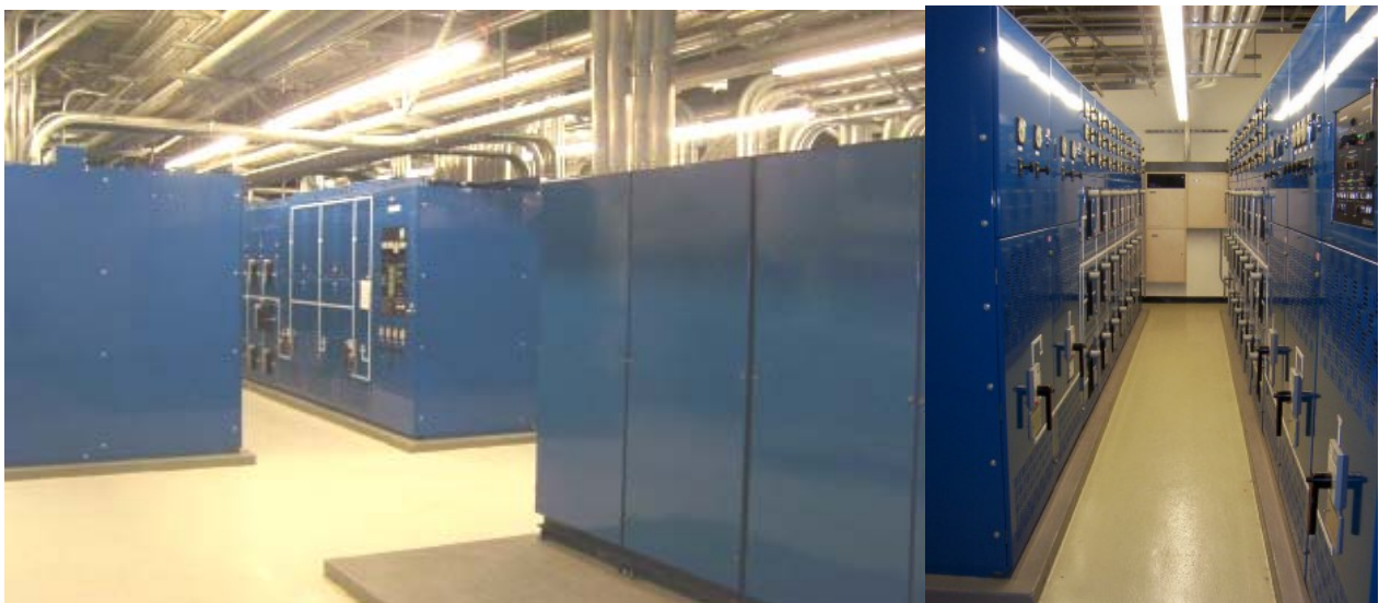
Existing UPS showing pad area for expansion to 5 th module on A & B systems
