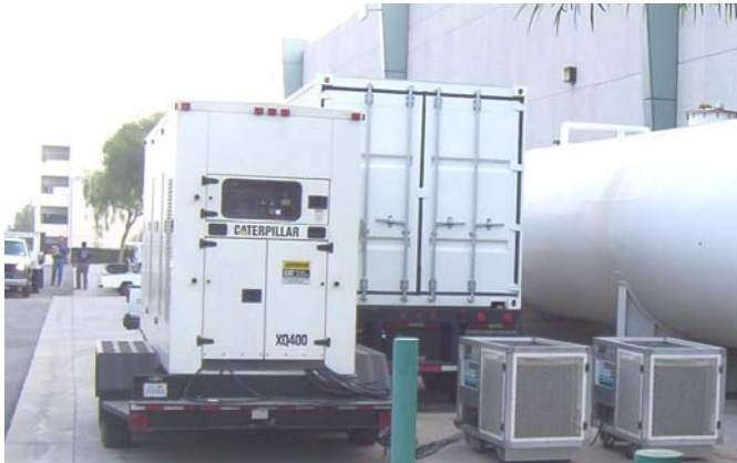
Roll-up UPS, dedicated Genset & support AC (1 of 2)
