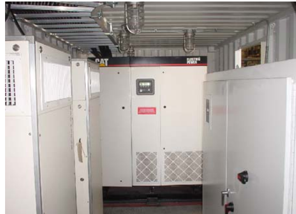
Interior of Roll-up UPS Module
