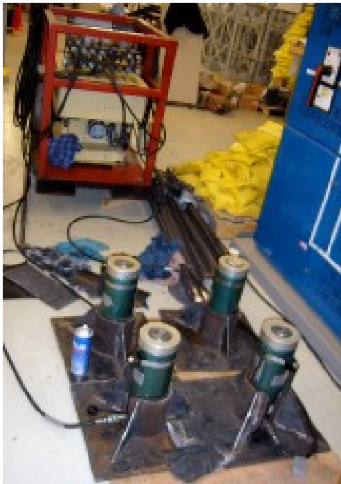
Manifolded Hydraulic Lift System
