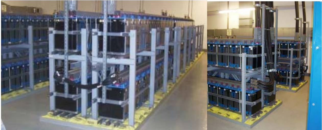
Main UPS Battery Room – before reinforcement
