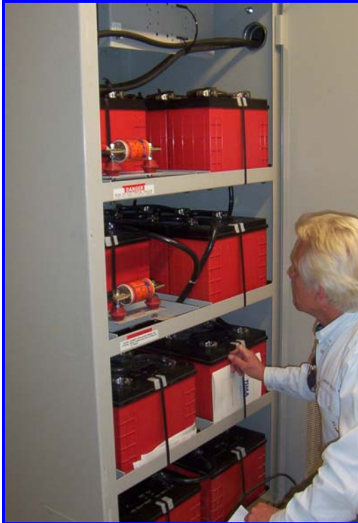
Fig. 2a 3-5 yr VRLA batteries in cabinets
