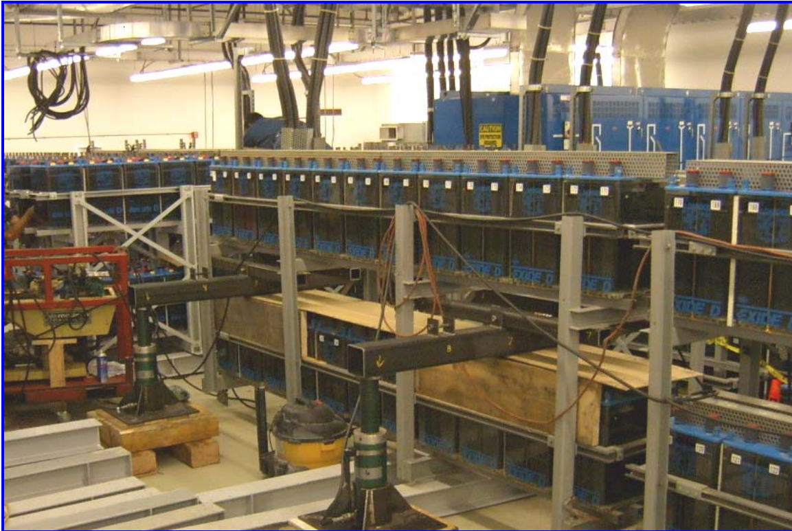
Fig 1. A very unique project, this client required massive above slab reinforcement to accommodate the weight of a flooded battery addition to its existing UPS battery room.
