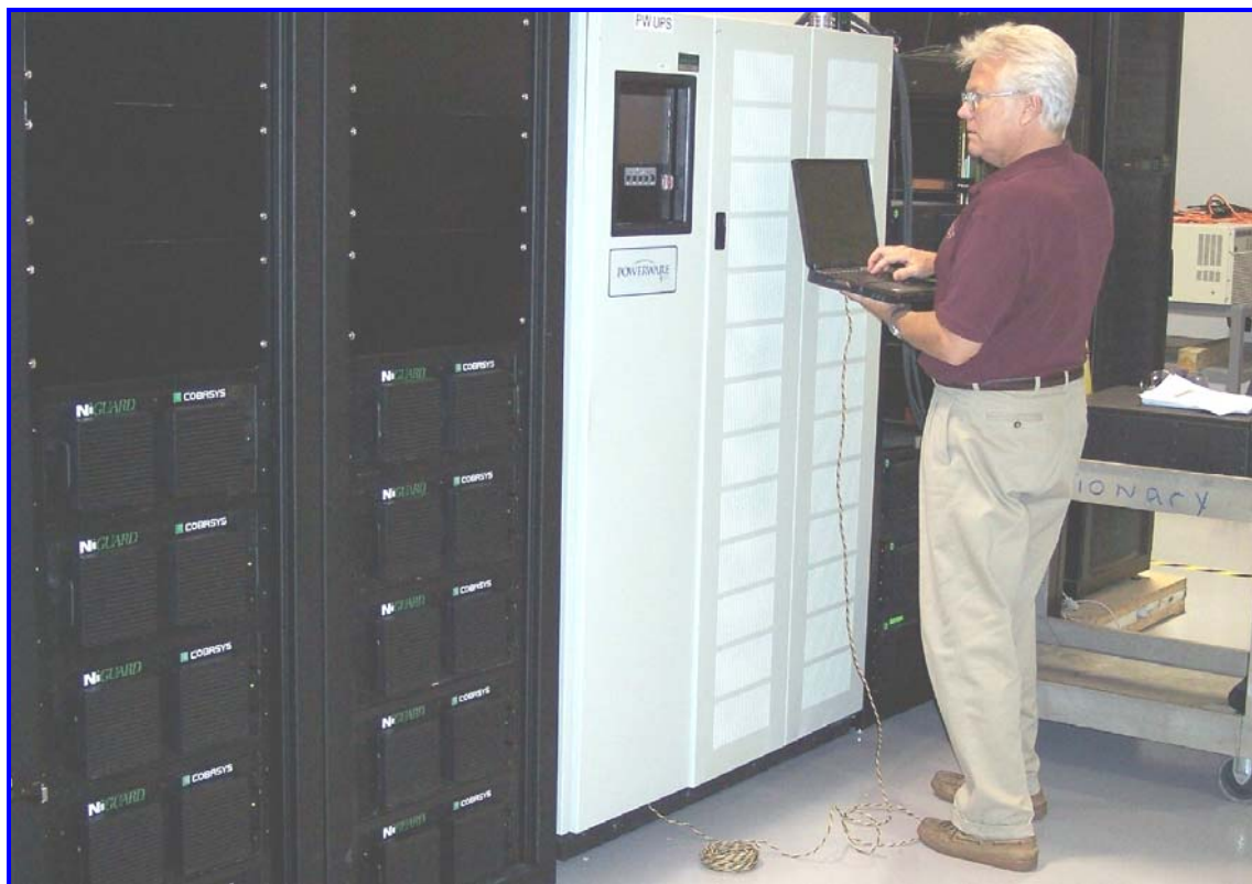
Fig.6 Author performing cycle testing on Powerware 9315 UPS w/ 15 minute NiMH battery
